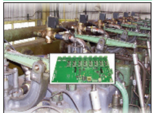
AutoBalance™ system installed on a Clark HBA-8T (turbocharged)
